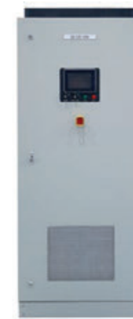
Power Conditioning System
