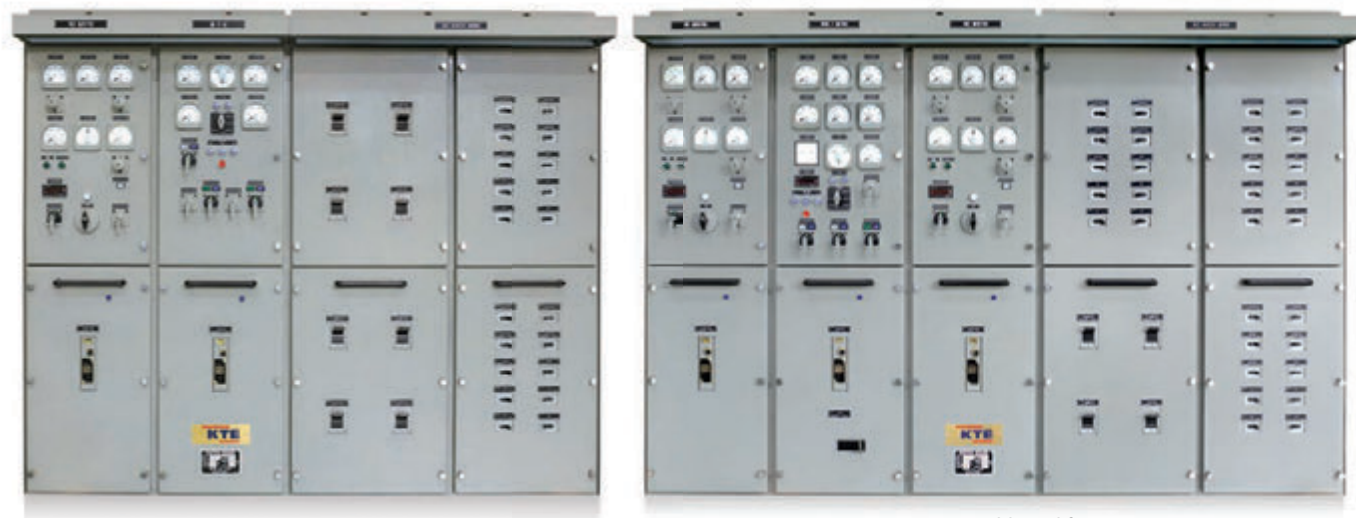
Main Switchboard for MSH(Mine Sweep Hunter)
